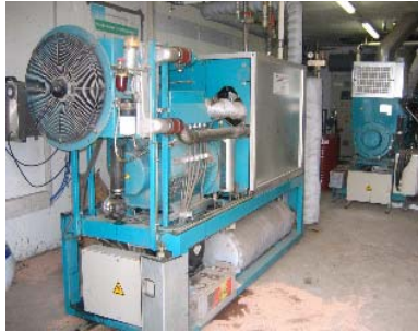
A biogas plant in Germany.
